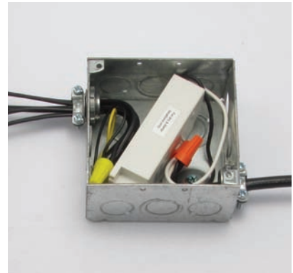
Tivoli 20 watt 12VDC power supply in 2 gang box
